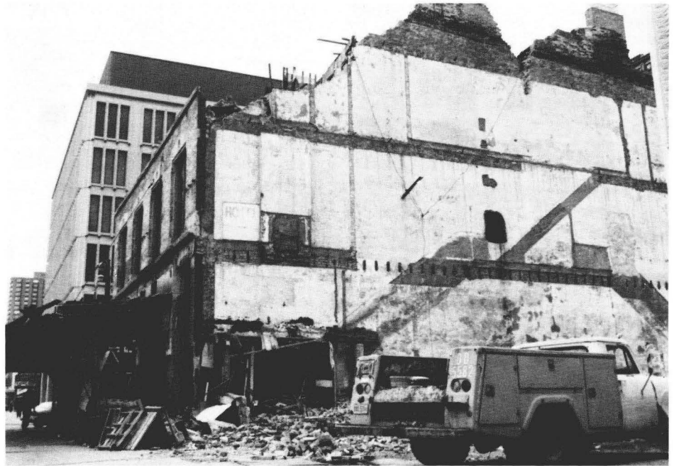
The destruction of a South Loop SRO.
